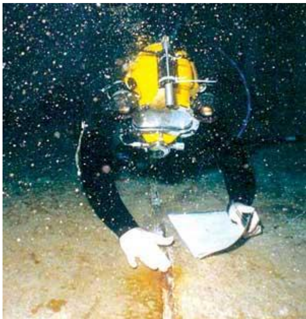
At D'Arbonne Dam, divers used information gleaned from the use of acoustic imaging and profiling to pinpoint specifically where underwater repair work was needed.
