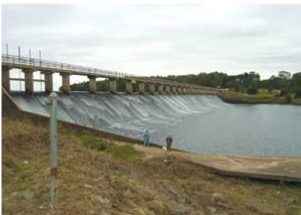
Using underwater acoustic imaging and profiling at the 50-year-old D'Arbonne Dam in Louisiana, contractors generated a detailed model of sub-surface conditions. This model verified the presence of voids under the spillway apron; repair is nearing completion.
