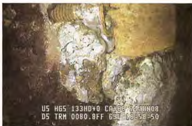
Above and below: Images from the ROV show the substantial damage
