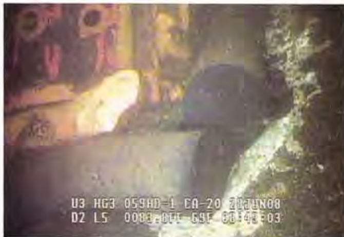
The gate did substantial damage to the concrete base of the scroll case
